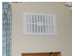
Typical controllable background vent in
