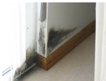
Lack of adequate ventilation can lead to mould growth due to condensation
